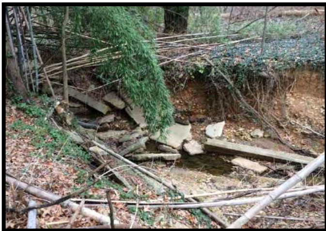
FIGURE 7: Bank erosion, concrete, and bamboo
