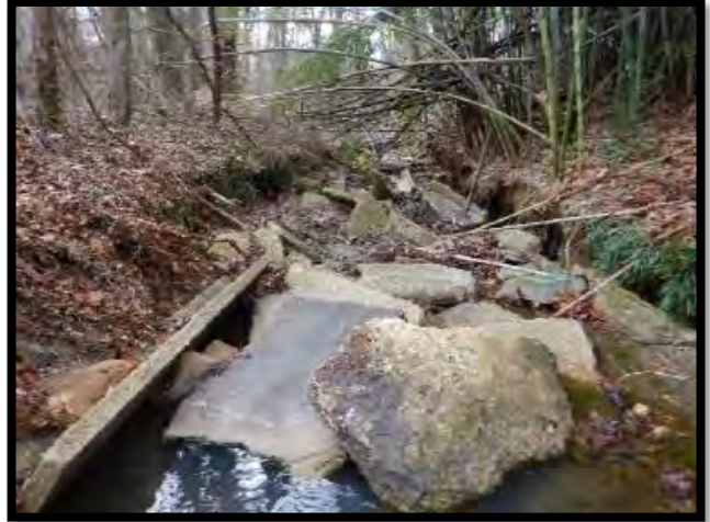
FIGURE 3: Bamboo and channel debris blockage in
