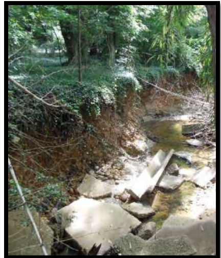
FIGURE 6: Bank erosion, concrete and bamboo
